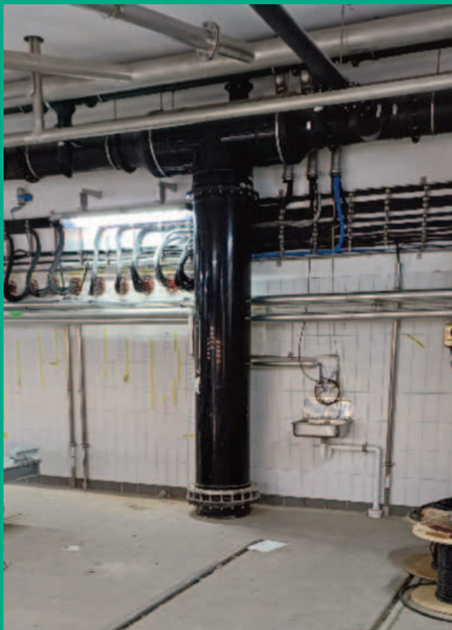
pipng inside building
