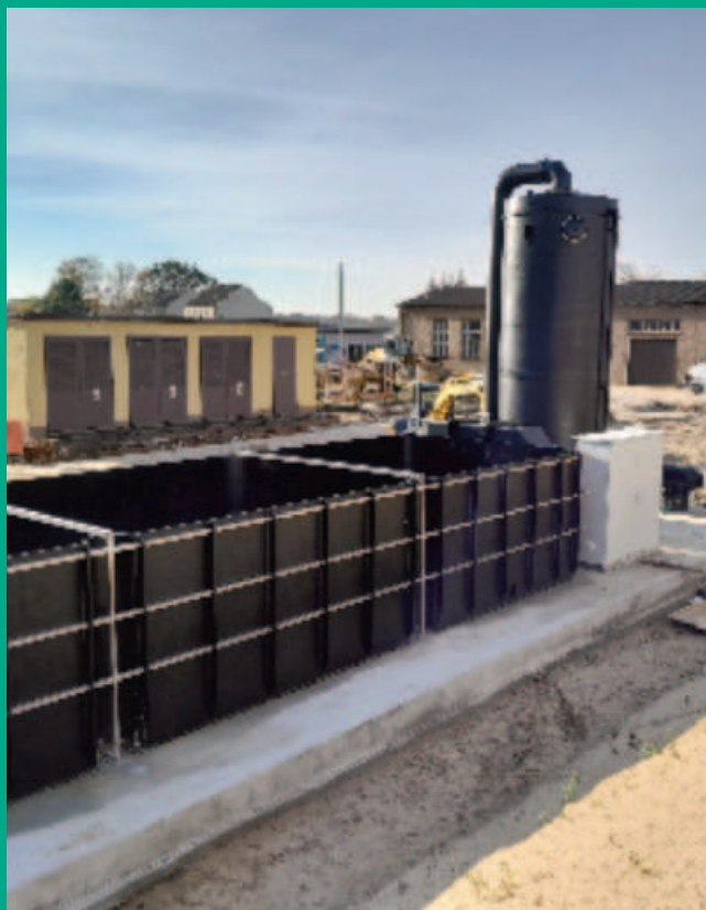
exhaust air treatment system with control cabinet
